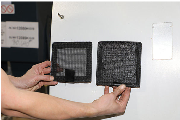
A dirty filter (right) can cause a machine's electrical cabinet to overheat. (Image provided by Absolute Machine Tools)
